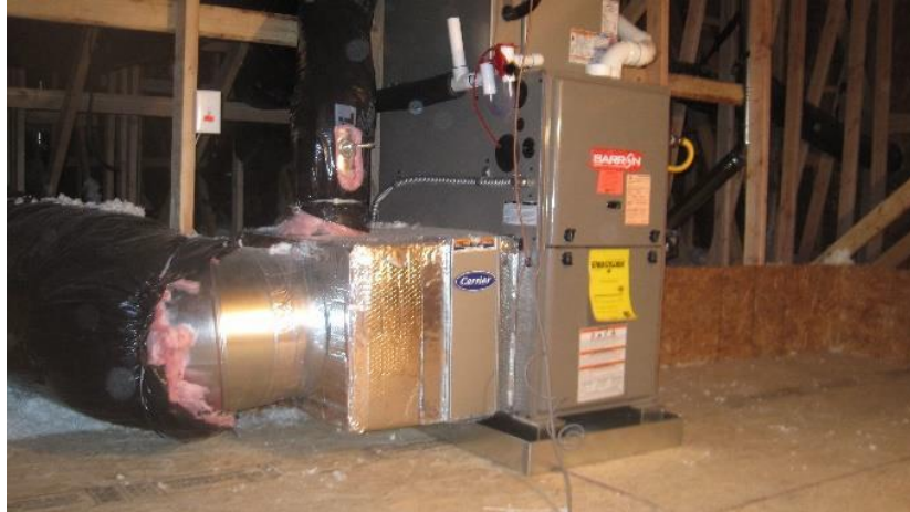
Figure 46: DU 1.3 Duct Insulation and Duct Seal
