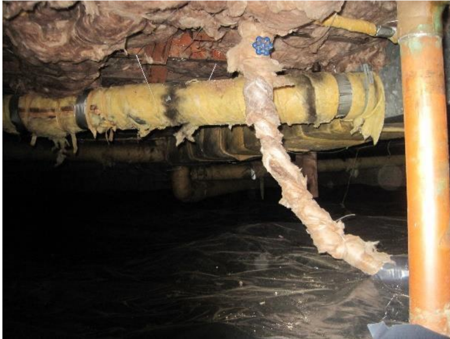
Figure 43: DU 1.7 Leaky duct showing dirty insulation where sealing is missing
