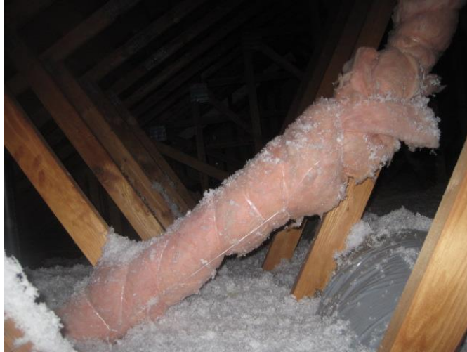
Figure 47: DU 1.4.1 Correctly Insulated Exhaust Vent
