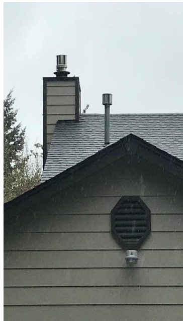
Figure 23: VE 1.5 Exhaust Vents
