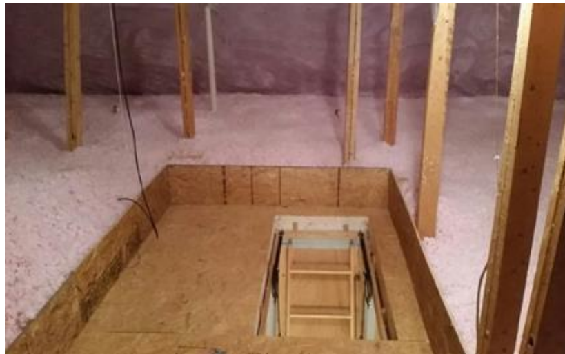
Figure 5: PR 1.3.2 Attic Access damming
