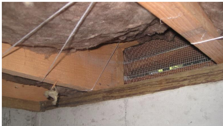
Figure 22: VE 1.5 Crawlspace Ventilation
