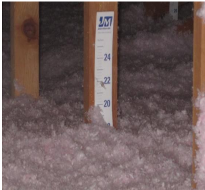
Figure 12: AT 2.2.1 Insulation Marker
