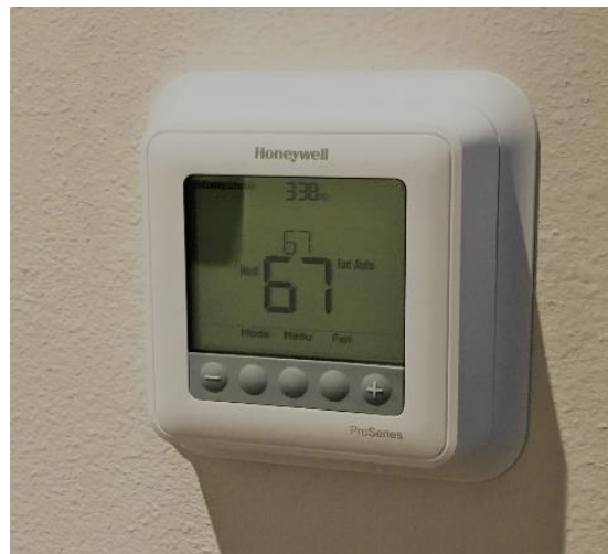
Figure 56: PT 1.1 Honeywell Programmable Thermostat
