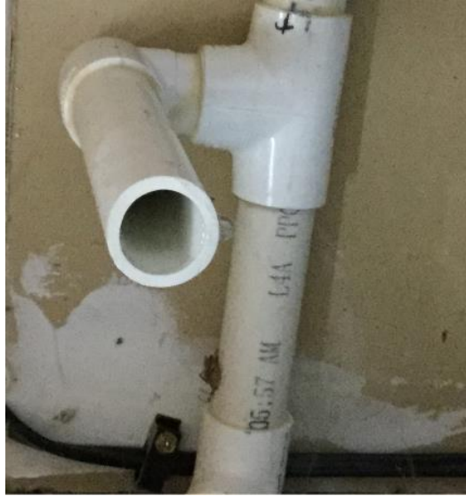
Figure 52: BO 1.0 Secondary condensate drain
