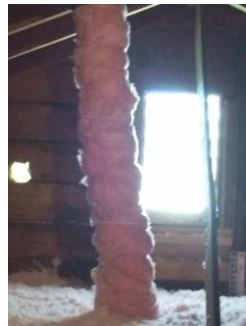
Figure 21: VE 1.2 Insulated Exhaust Vents to the Outside
