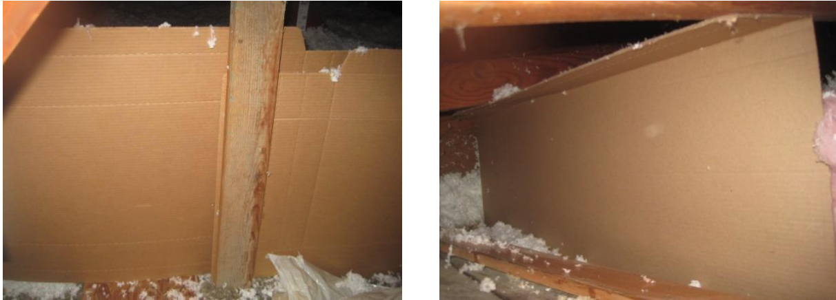
Figure 6: PR 1.3.3 Damming in Attics
