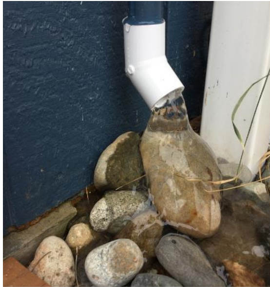
Figure 51: GF 1.2 Ice Dam at Condensate Termination
