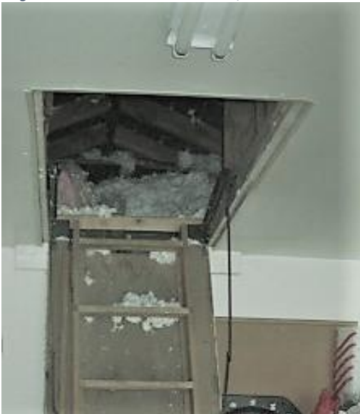
Figure 10: AT 1.1.1.1 Attic Access w/ Insulation leak
